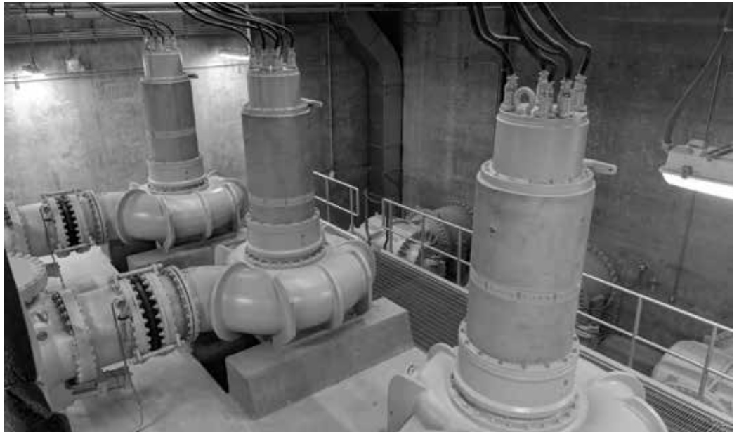
At 30 feet below ground, this reinforced concrete chamber houses the pumps and equipment vital to flood protection measures for The Ohio State University's extensive medical campus infrastructure located near the Olentangy River.
