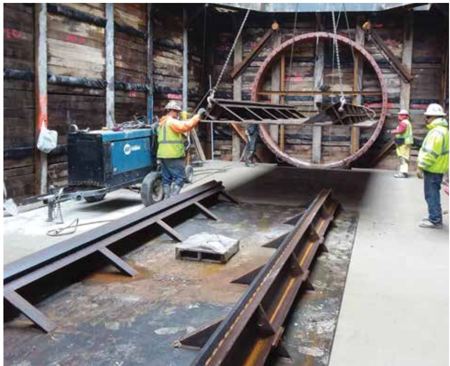
Launch frame being installed. This 4.5 mile stretch of sanitary interceptor sewer extends from south of Blacklick Ridge Boulevard to Morse Road and services approximately 16,000 acres within the Blacklick Creek watershed.
